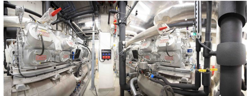
Heat pump system at the Therme Wien spa © Klimafonds/Krobath
